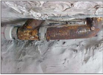
This badly corroded cast-iron lateral was typical of the sewer pipes under Darcy Hall before rehabilitation.
