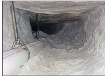
Workers inserted anchors, then threaded in hangers to support the Schedule 40 PVC replacement pipe.
